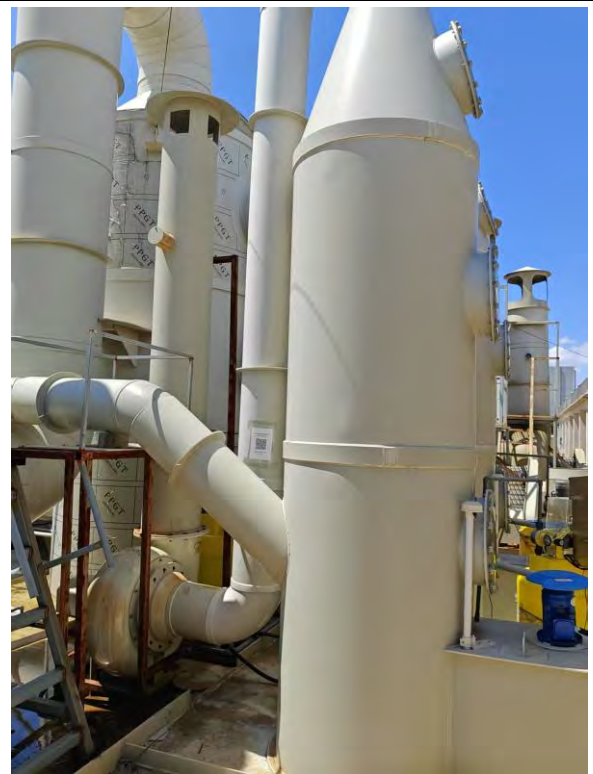
DA011/三层喷淋塔
