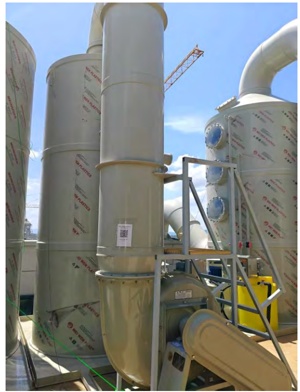
DA009/三层喷淋塔
