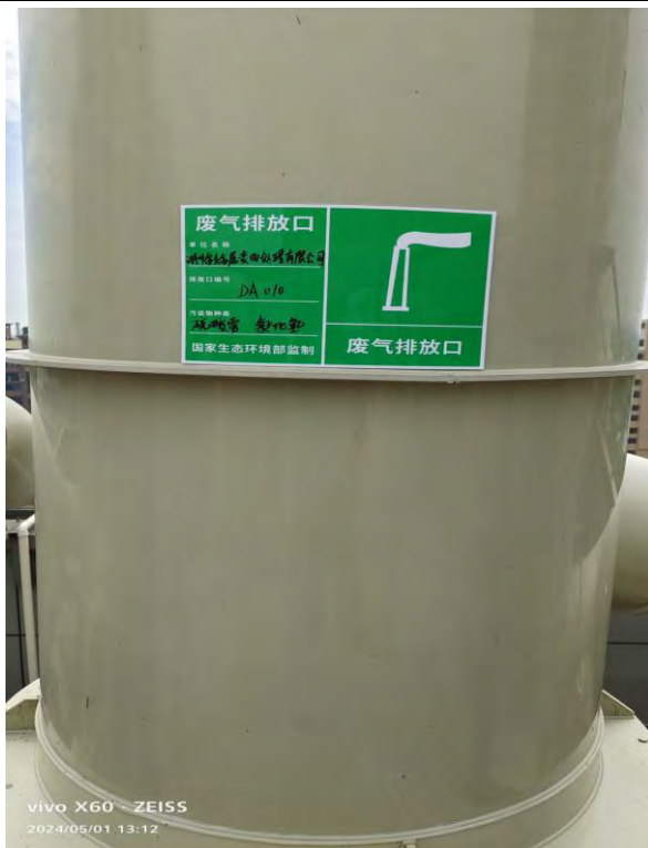
DA010/三层喷淋塔
