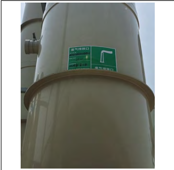
DA001/三层喷淋塔
